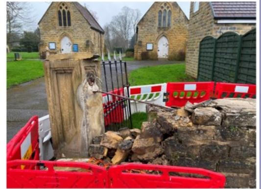
Church on Corner Damage from in March 24 - No Mention in any Meeting Minutes
